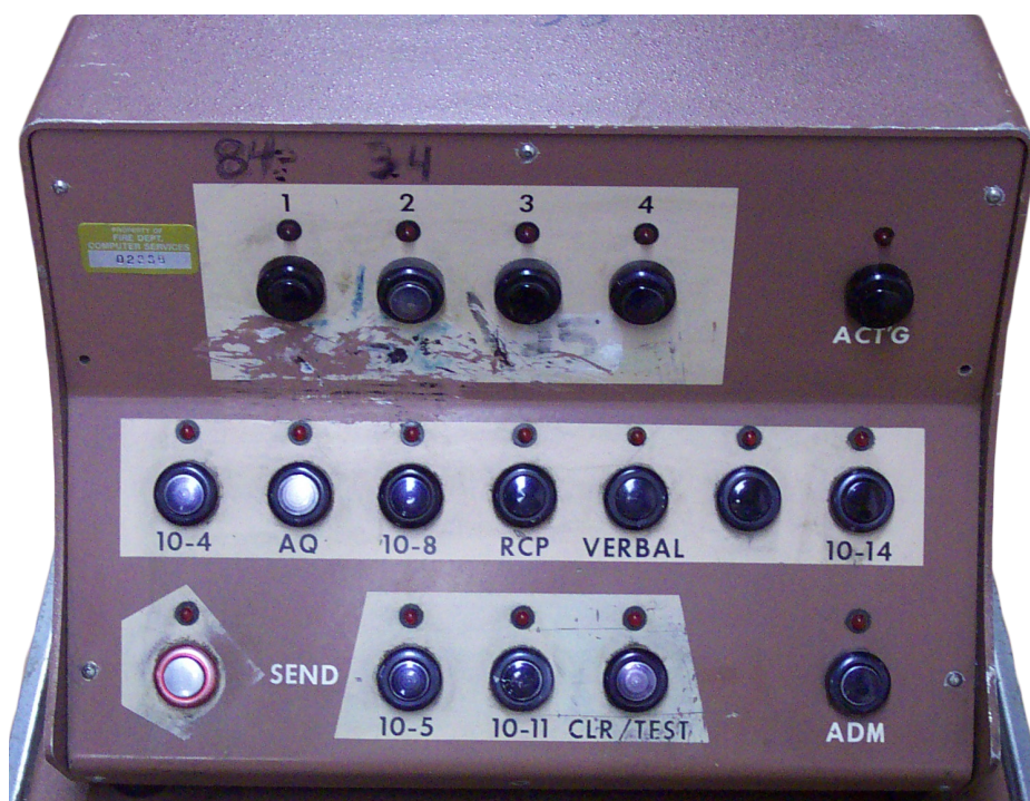
Figure 10 Alarm Teleprinter/Selector (Kevin Jones)
